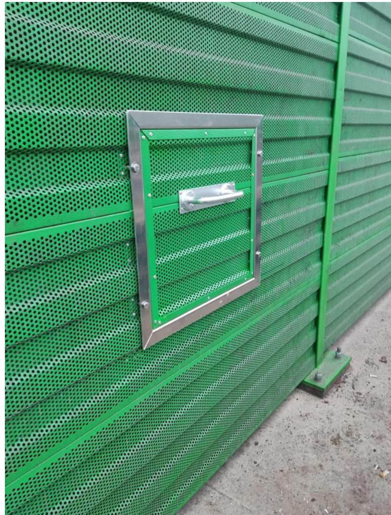
Photo 14. Photo of a point inspection hole used to check devices monitoring the tension force in nails
