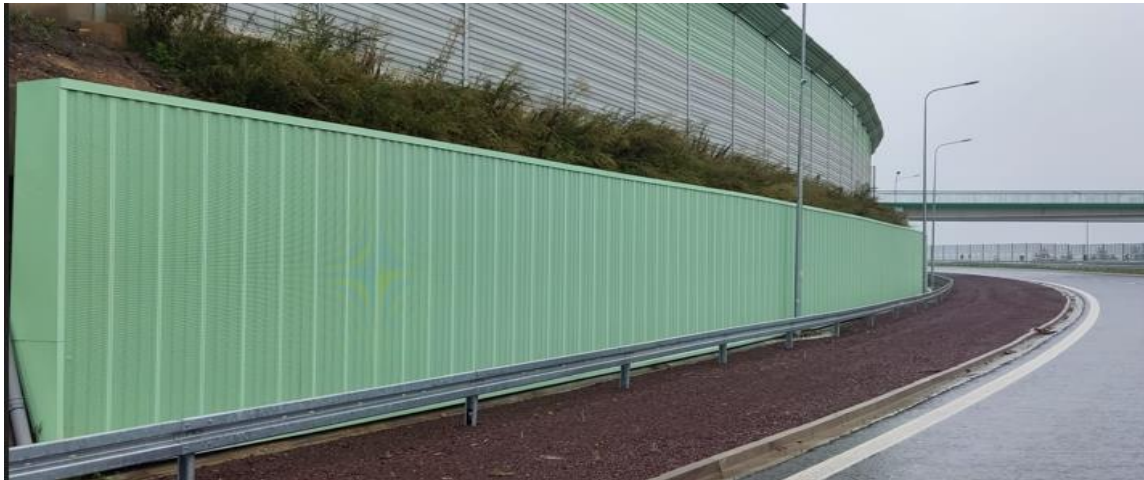
Photo.2. Photo after the palisade facing for the project titled: "Construction of the bypass of the city of Wałbrzych along national road No. 35 from km 2+350 to km 8+250"
