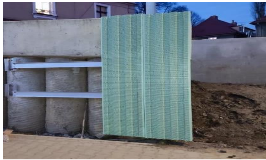
Photo 6. Execution of the substructure for the palisade facing at the implementation stage for the task titled "Construction of the bypass of the city of Wałbrzych along national road No. 35 from km 2+350 to km 8+250"
