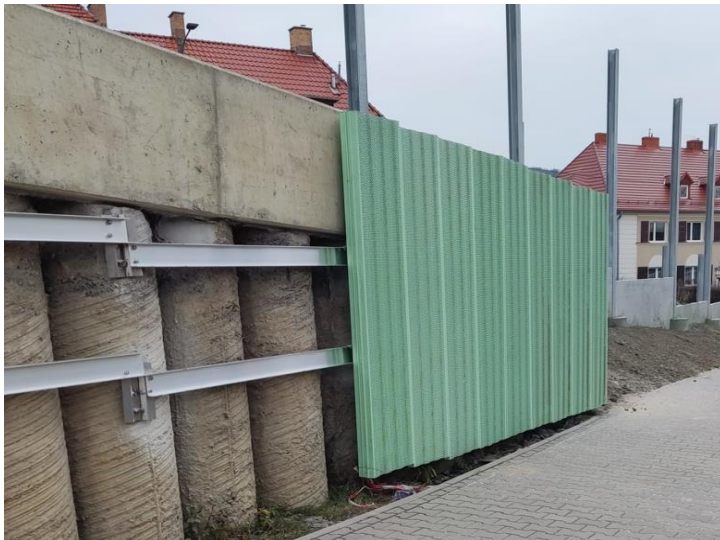
Photo 5. Execution of the substructure for the palisade facing at the implementation stage for the task titled "Construction of the bypass of the city of Wałbrzych along national road No. 35 from km 2+350 to km 8+250"
